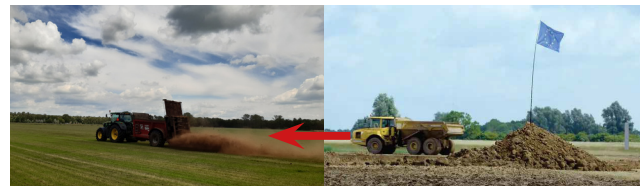
The pictures depict freshly excavated clay from a floodplain where space is made for flood alleviation (right) and drought-prone sandy soil where this clay finds a new use (left).
