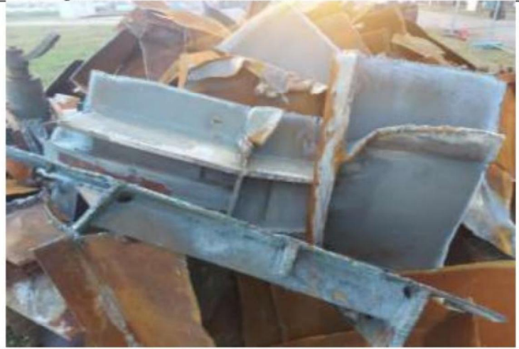
Description photo: 26-2-2021 metal pieces outside the fencing after removal asbestos
