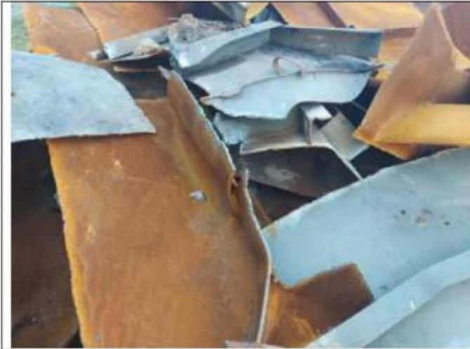
Description photo: 26-2-2021 metal pieces outside the fencing after removal asbestos
