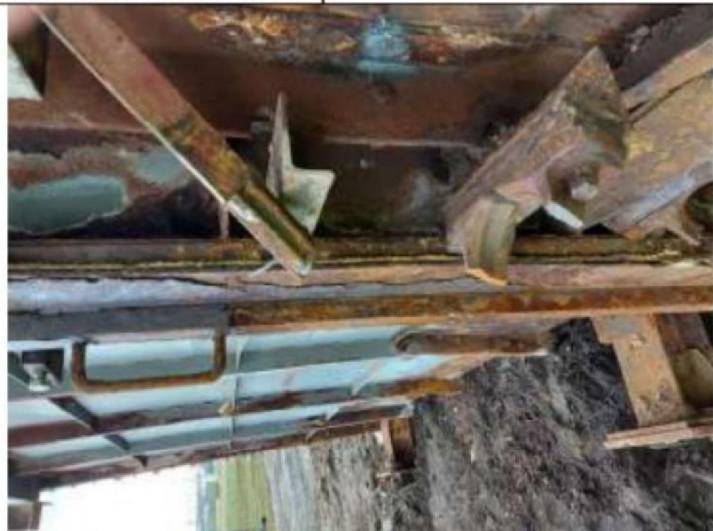
Description photo: 26-3-2021 parts off separation between FGD and Precips. This parts includes textile bandage which has to be separated.
